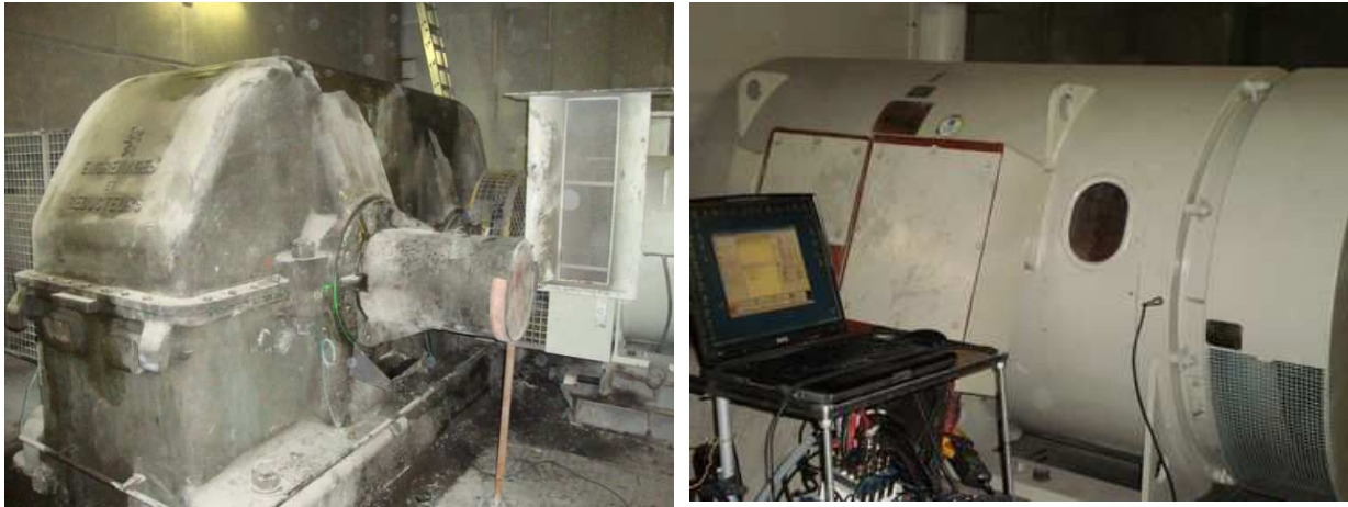
Fig.2 : reduction gearbox and motor driving a ball mill
